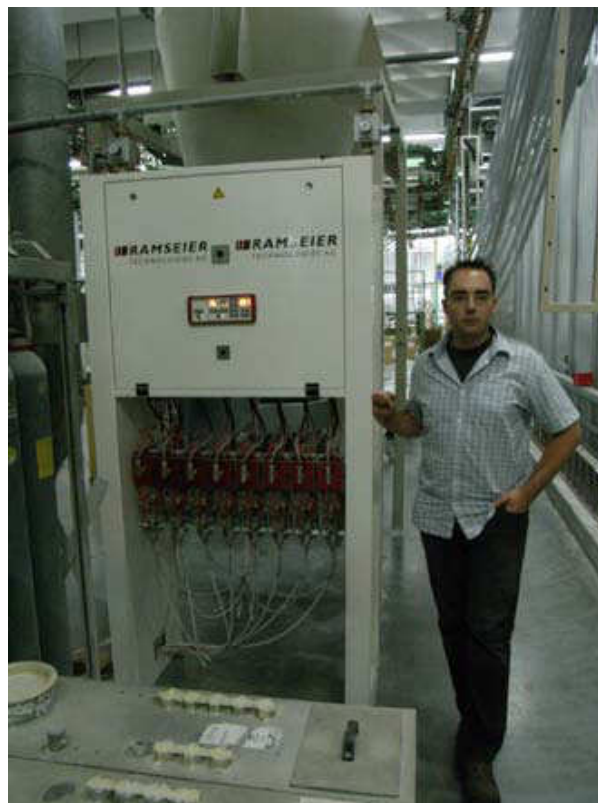
▲coating director Patrick Witzgall, after the first months of the refurbished facility very satisfied by up to 20 percent of the powder decreased consumption.
